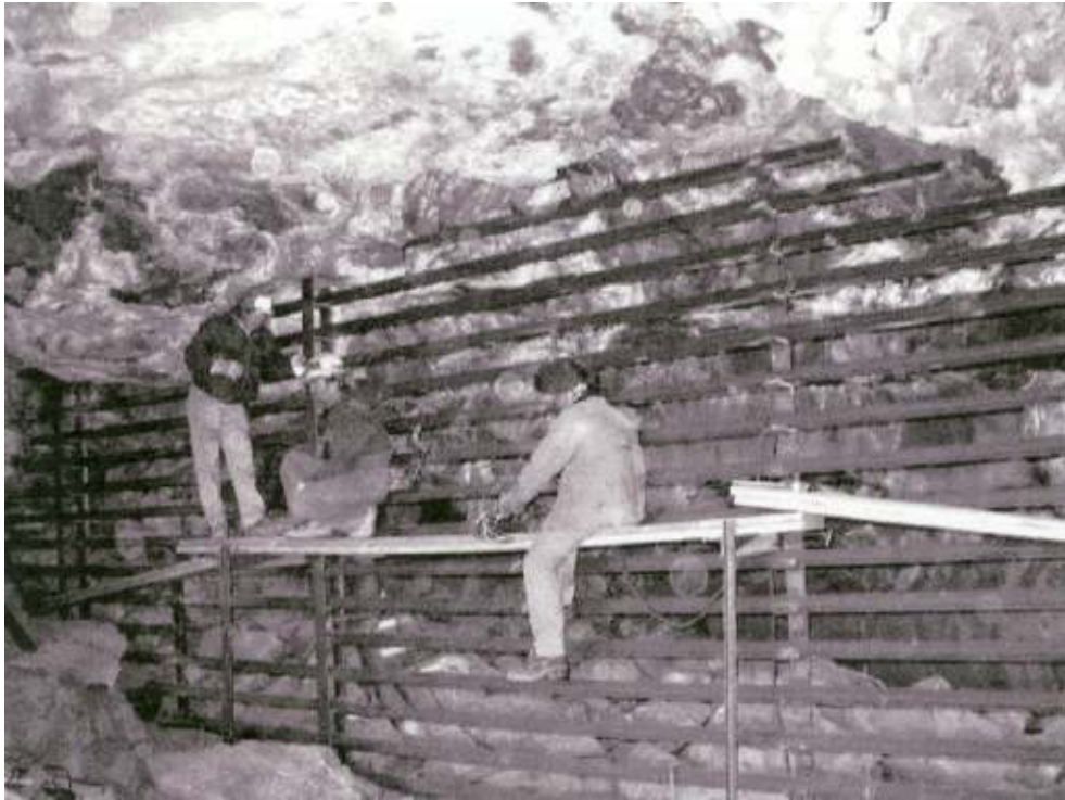
Scaffolding was needed to work on the upper portion of the gate. 9-00.
