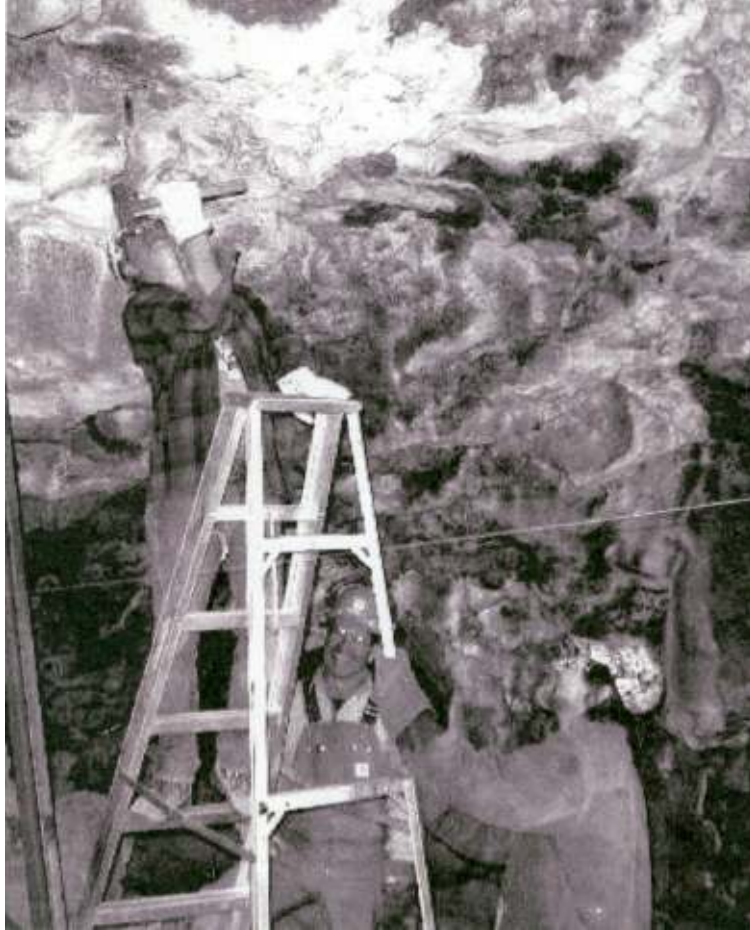
Bill Kenney stabilizes a ladder as the ceiling is prepped for the uprights. 9-00.
